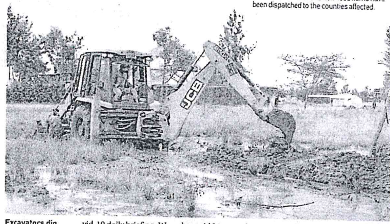
Excavators dig trenches at Mugutha village in Juja, Kiambu county. Residents are racing against time to clear waterways. PO/ MATHEW NDUNGU
