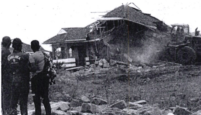
A bulldozer demolishes a house on land that belongs to the East African Portland Cement Company in Athi River on Monday. [Peterson Gitthaiga, Standard]
