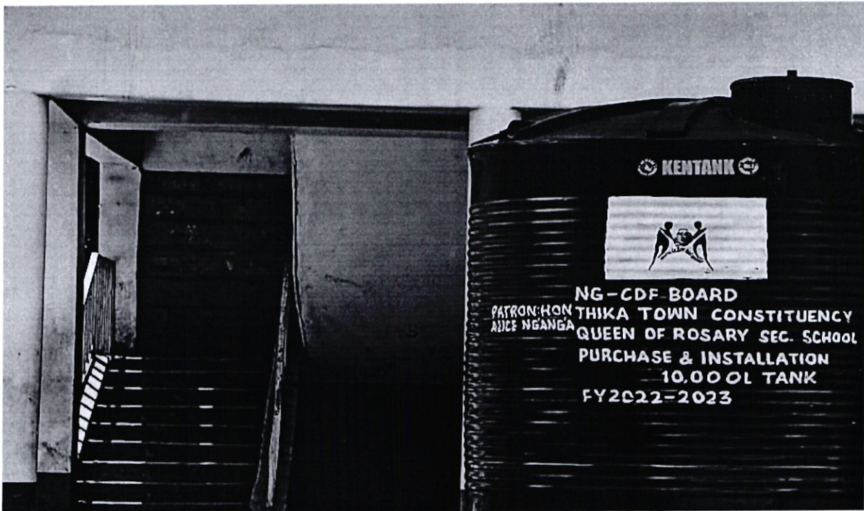
Supply and installation of 10,000l water tank on a Concrete base platform at Queen of Rosary Secondary School (Environment)
