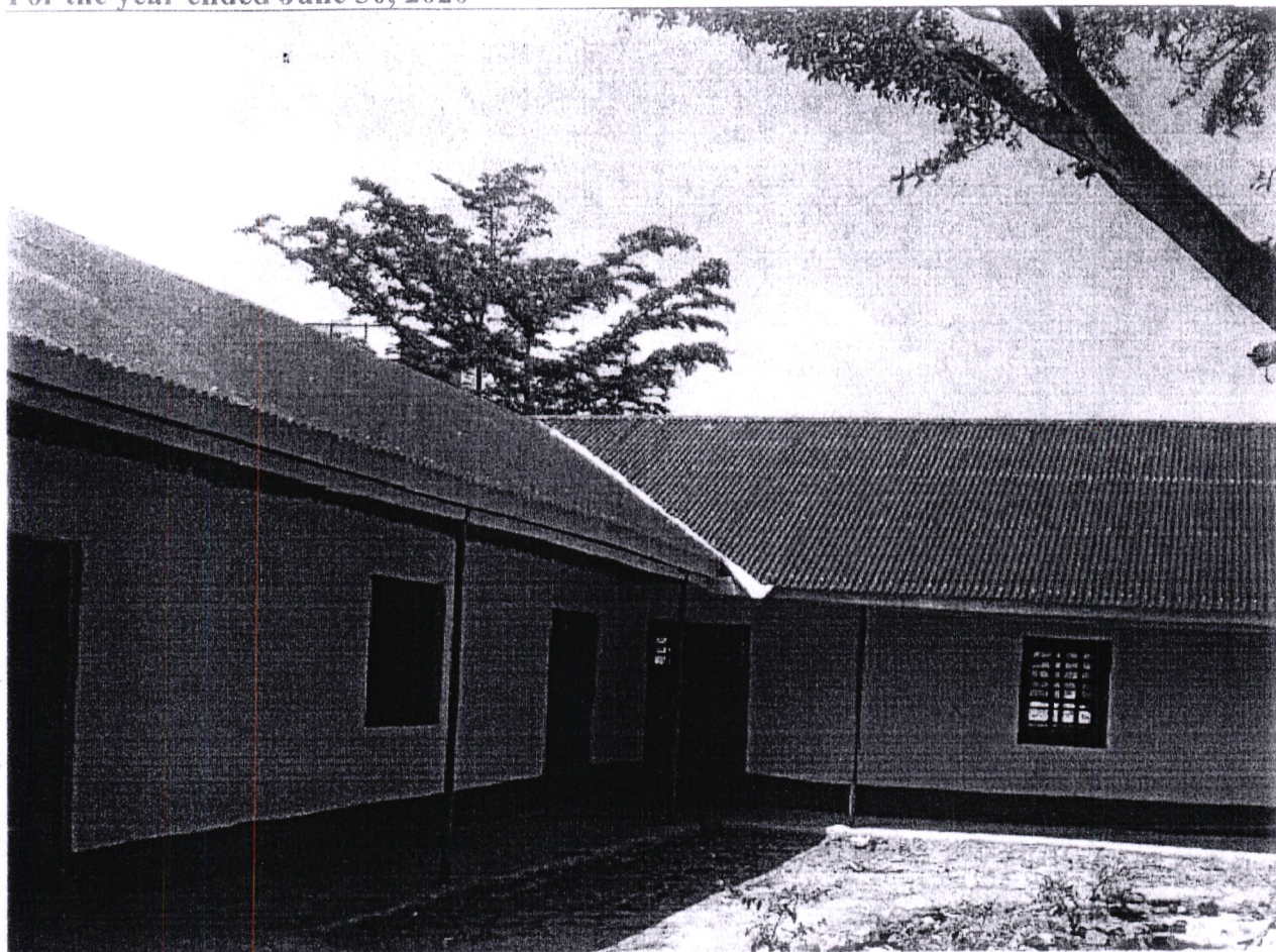
RENOVATION OF FOUR CLASSROOMS AT MALELE PRIMARY SCHOOL FUNDED BY GEM NG-CDF FY 2019/2020
